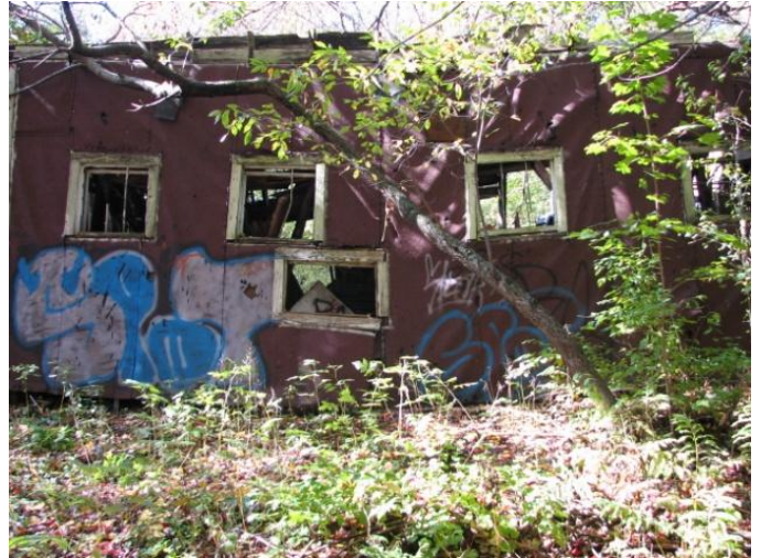
Photo 2. Decrepit shed on south side of the property is a safety hazard and should be removed.
