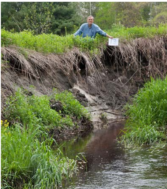
Bank erosion on a stretch of Vine Brook.
