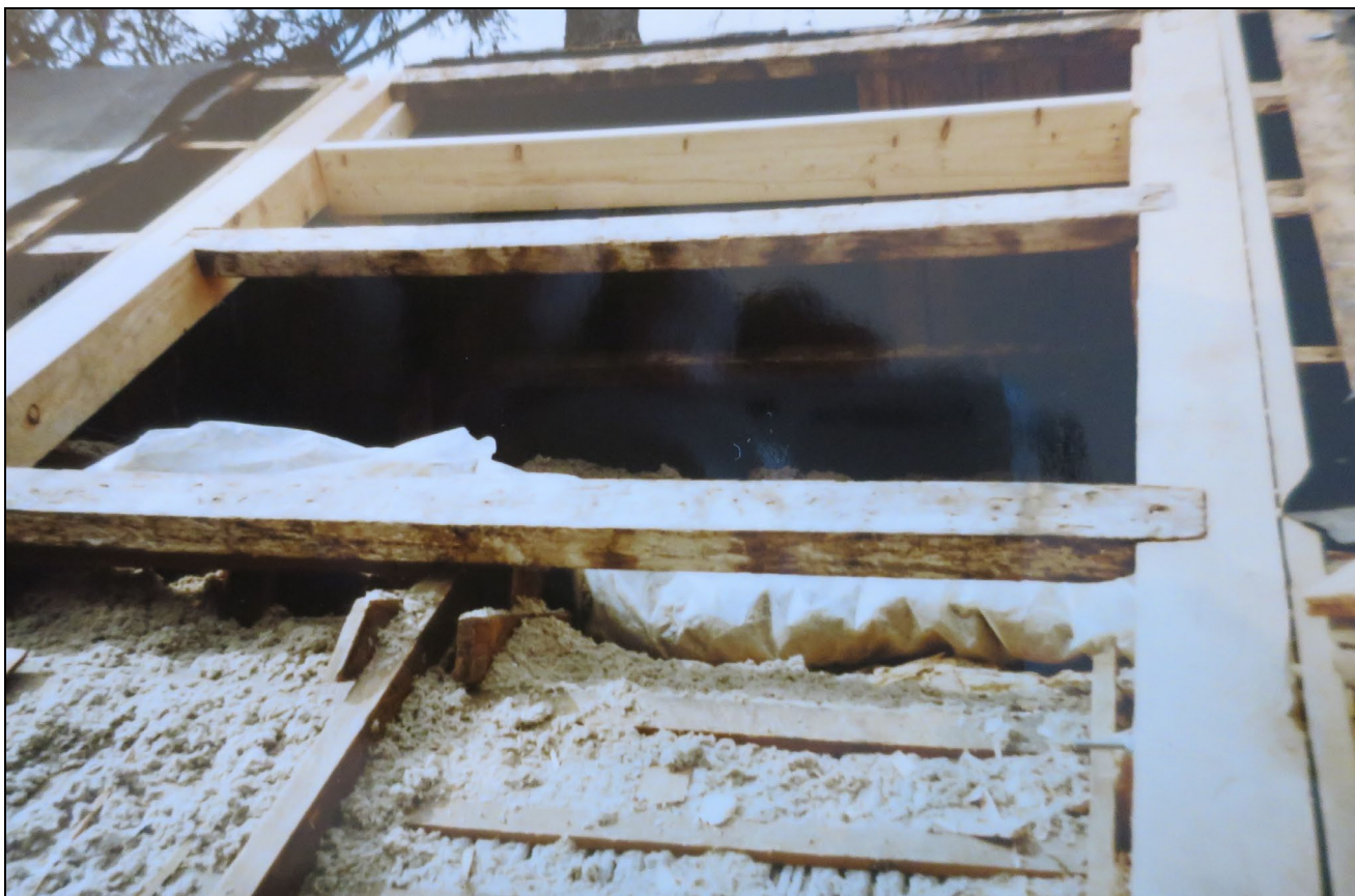
Fig.12: Photograph of roof repairs made in 2011 showing replacement of principal rafters on west side of house. Owner's collection.
