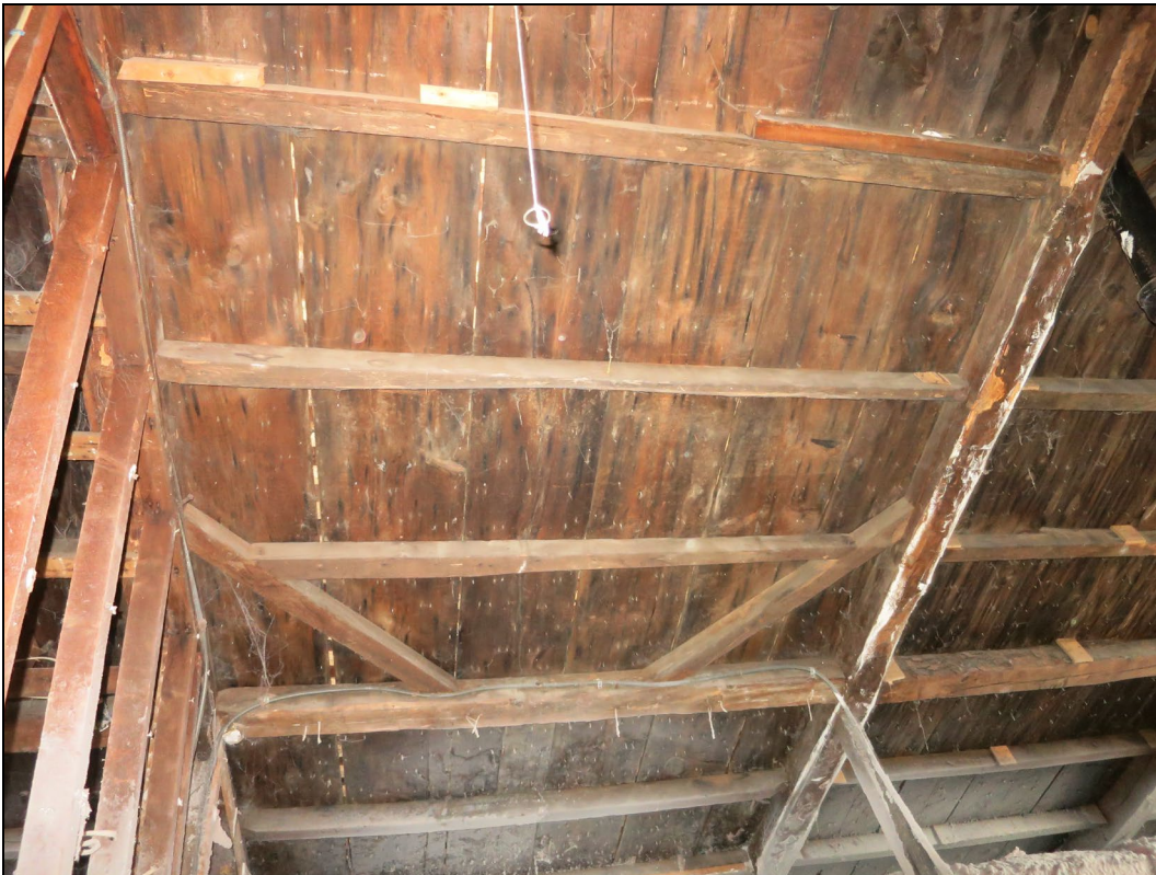
Attic, detail of roof framing, north side, showing large purlin and bracing.
