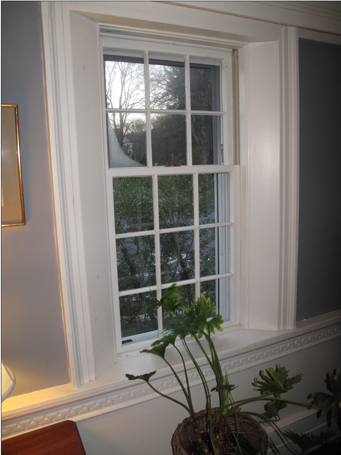
First floor west parlor, window in west wall showing beveled window reveals and carved chairrail with meander pattern.
